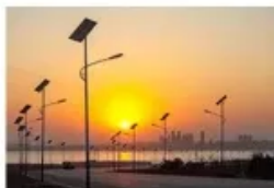
Solar Street Light
