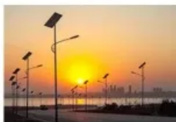
Solar Street Light
